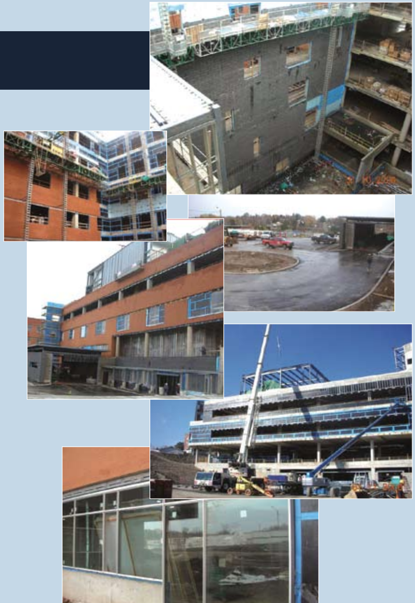
Clockwise from top: courtyard #2 being bricked; the newly paved ambulance entrance; erecting structural steel for WS level 6 penthouse; installing the first panes of glass in A2; a view of the north entrance; and a view of courtyard #5.
